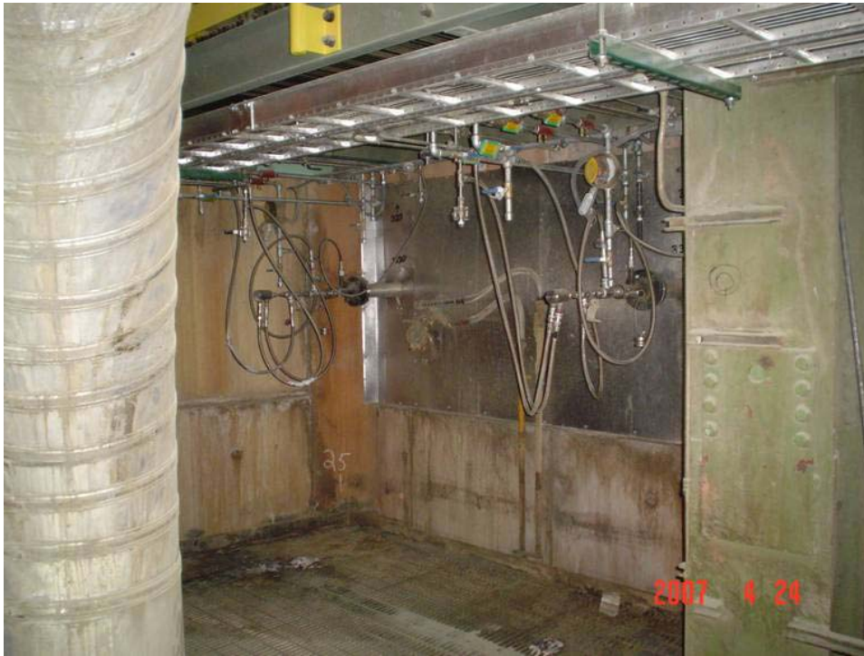
Figure 7. Two side-wall RRI injectors installed in Sioux Unit 2.
