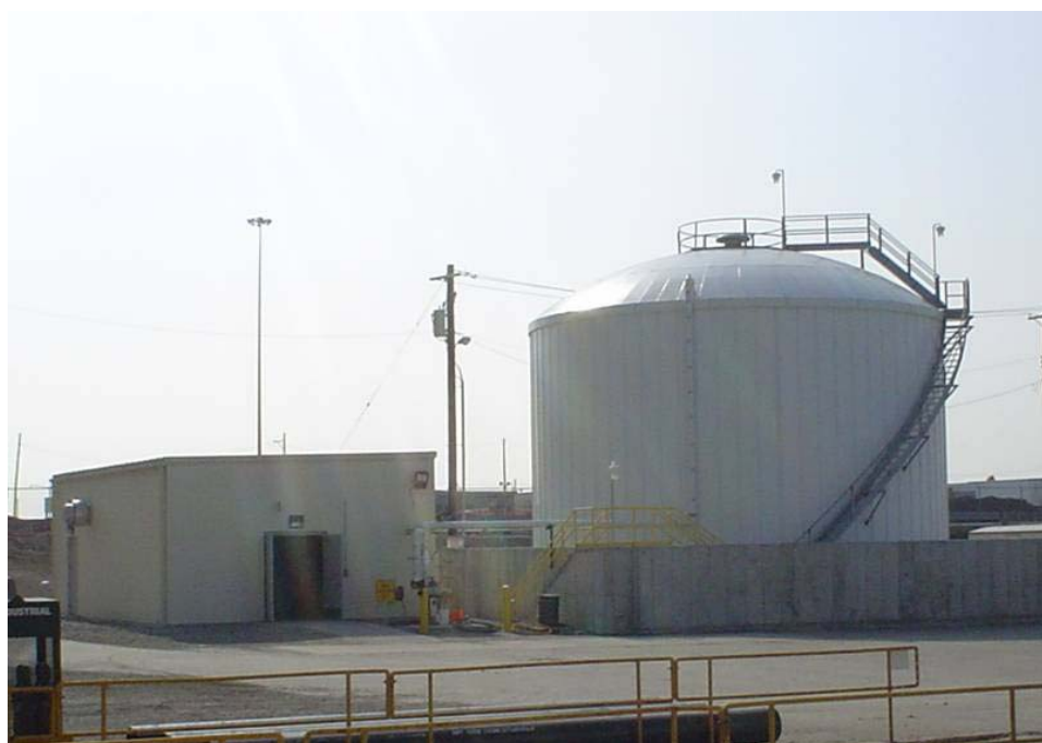
Figure 4. 400,000 gallon aqueous urea supply tank and adjacent pump house for the ALTA system at Sioux Plant.
