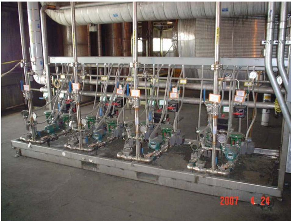
Figure 6. One of two FTI injection zone modules (IZM) where dilution water and aqueous urea are metered and mixed.
