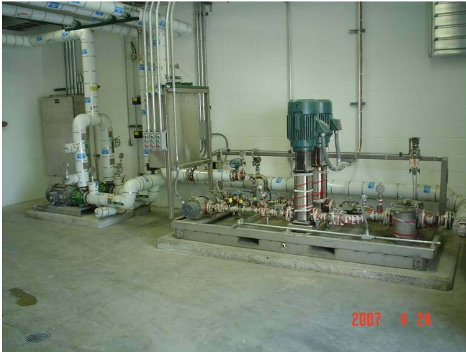
Figure 5. FTI's High flow delivery (HFD) pumps (center) and recirculation pumps (left) located inside the pump house adjacent to the urea storage tank.
